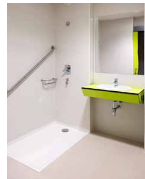
For interior finishes, all the floors were done in large-size porcelain stoneware tiles, and the same pieces were used for the protective skirting. The requirements for easy cleaning, aesthetic quality and durability were thus met. Above, the floors of the wet areas were done in Brown Avenue , 30 x 30 cm; and the walls,
